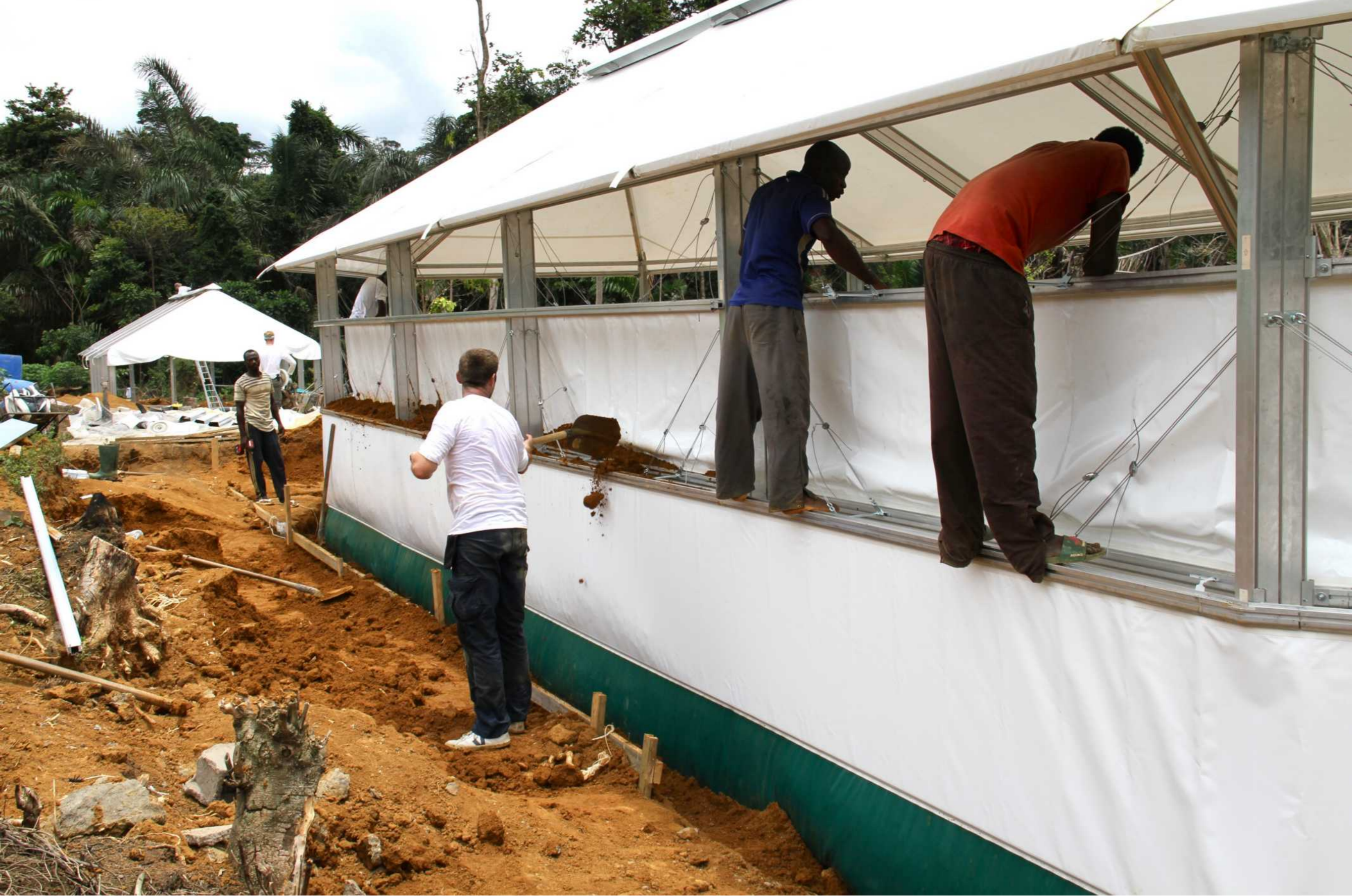
FILLING THE MAGGIE WALLS WITH 30 TONS OF CLAY GROUND THE TENT BECOMING A STURDY BUILDING
